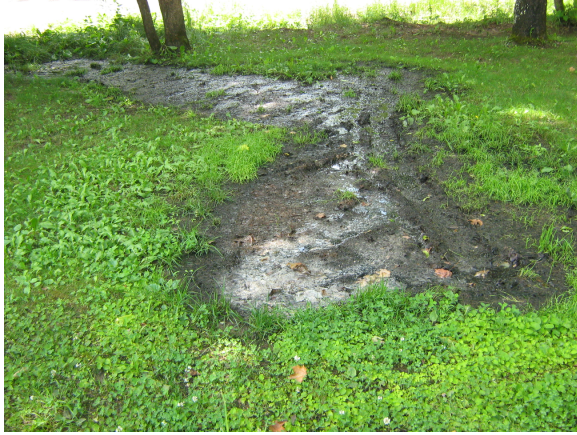
Figure 3. Example of a system that received a failed inspection [Photo credit: NBMCA]
