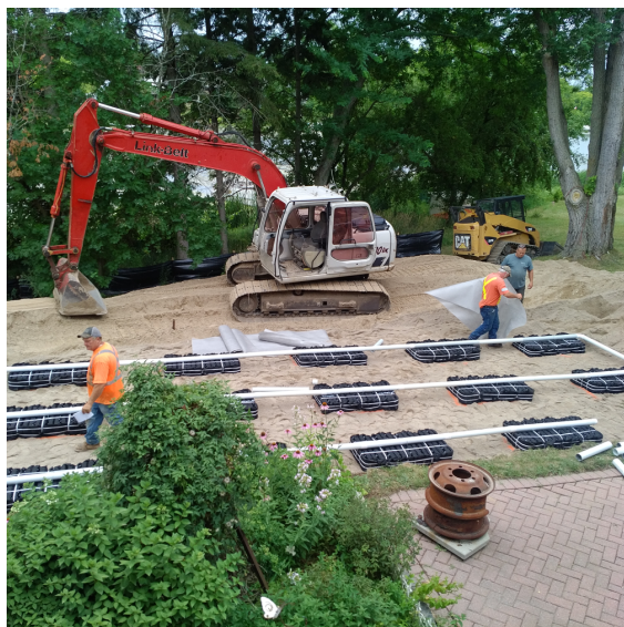
Figure 2. New Tertiary Septic System Installment Following a Failed Inspection of the Previous System [Photo Credit: Liz Huff]
